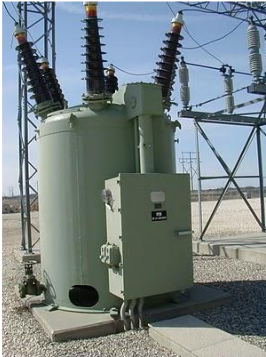
( b ) 66 KV circuit breaker
