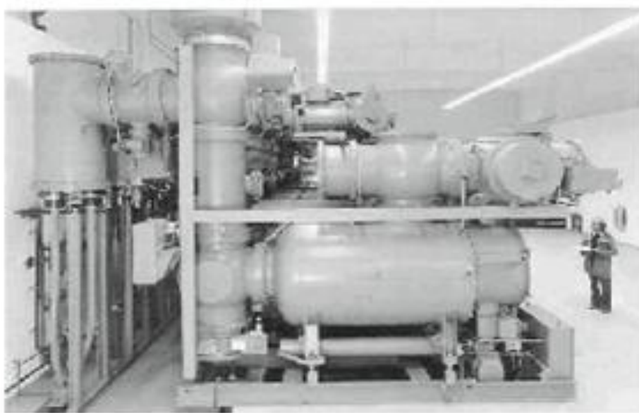
33 kV Indoor Type (GIS)
