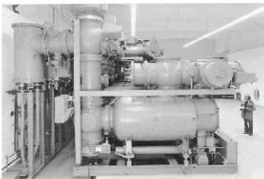
33 kV Indoor Type (GIS)
