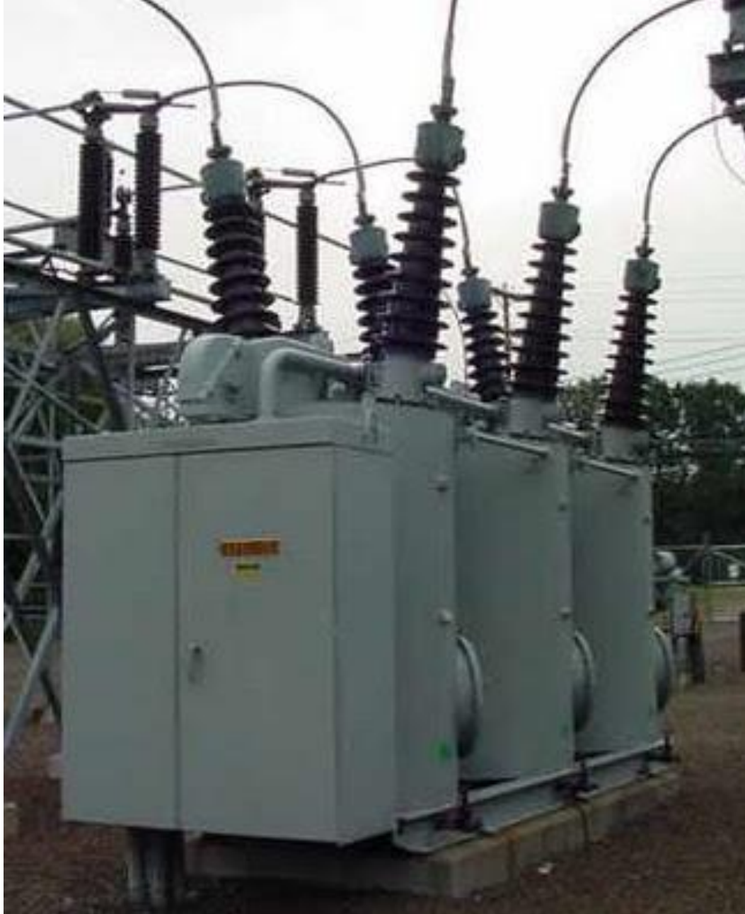
Prof. Dr. Sayed A. Ward (a) 115 KV circuit breaker C.Bs and Substations 4th Year Elec. Power Eng.
